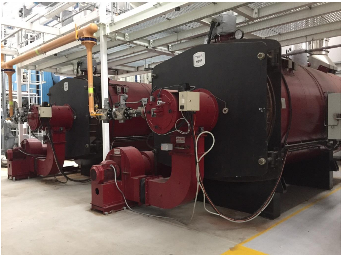
Picture: inside the Energy Centre at St Mary's
